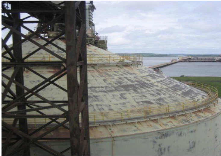
Figure 4: A photograph of the top of one of the Rusal Aughinish silos, with the conveyor belts going to and from ships in the background.
